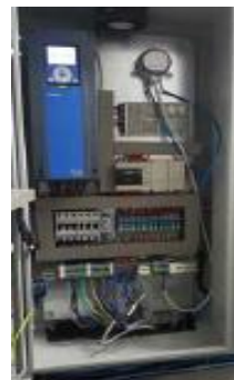
VSD & PLC Control
